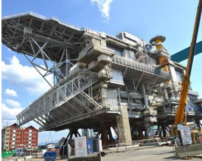
Johan Sverdrup utility and living quarter topside
